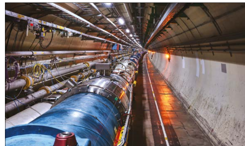
The LHC tunnel photographed in February.
