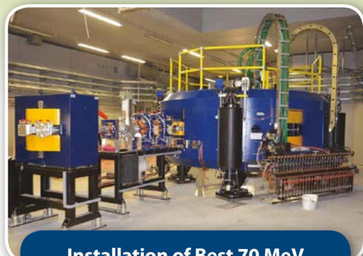
Installation of Best 70 MeV Cyclotron at Italian National Laboratories (INFN), Legnaro, IT
